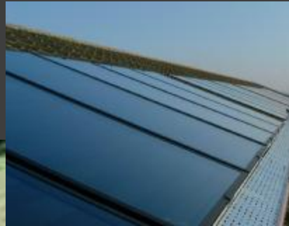
Solar thermal hot water
